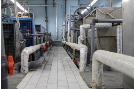
Insulated steam pipes
