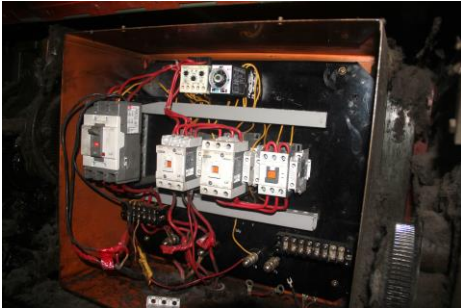
Star-delta drive installed on Ring Frame
